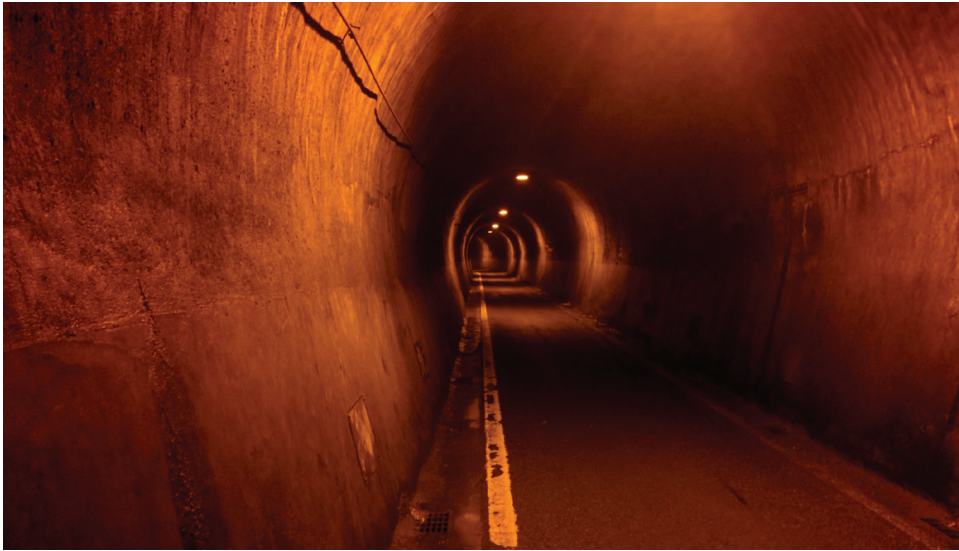
Figure 2. Inside Kiyotaki Tunnel, from the Kyoto side. Photograph by author. Click on the picture to experience going through Kiyotaki Tunnel in your browser.
